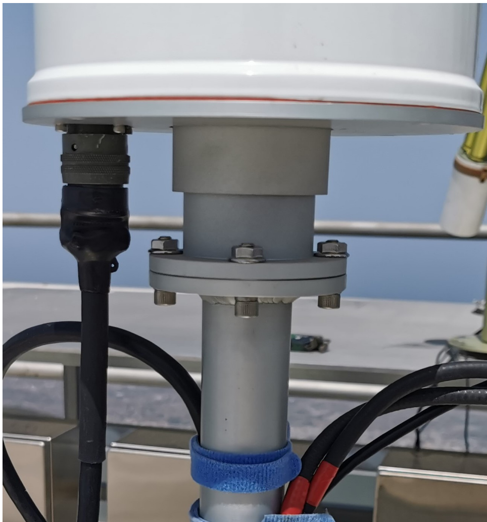
Figure 13: LuftBlick tracker TR1 - new vertical shaft
